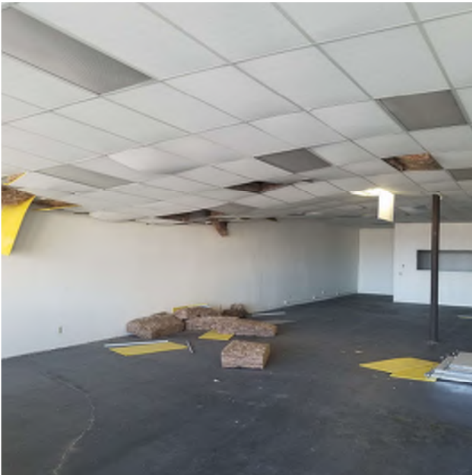
Photo O - Ceiling partially collapsed
