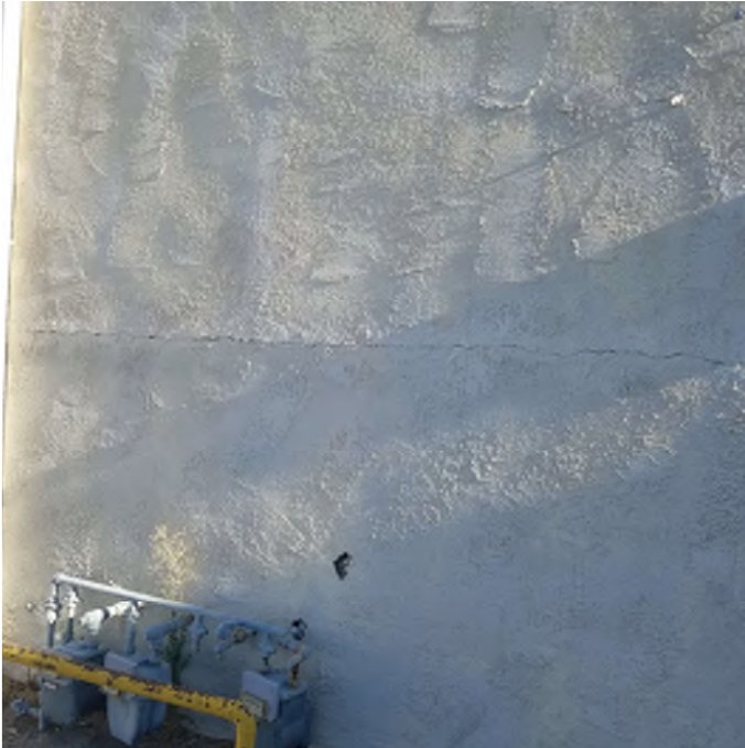
Photo M- Crack at back wall
