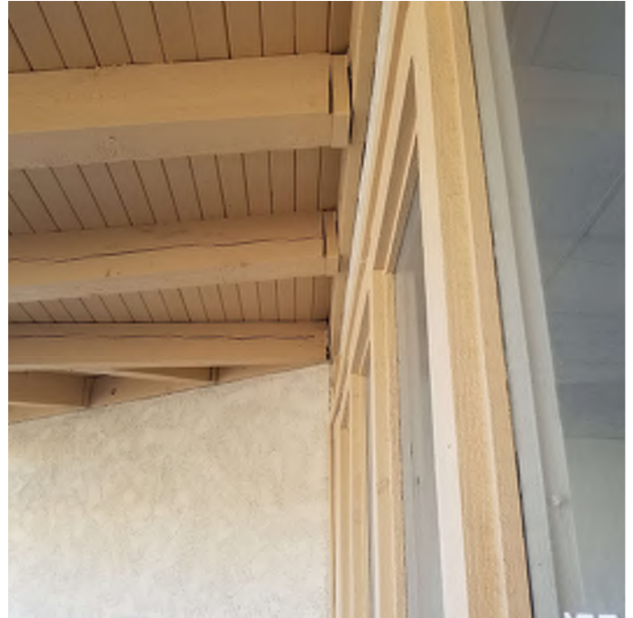
Photo R - Walkway cover beams pulling away from beam buckets
