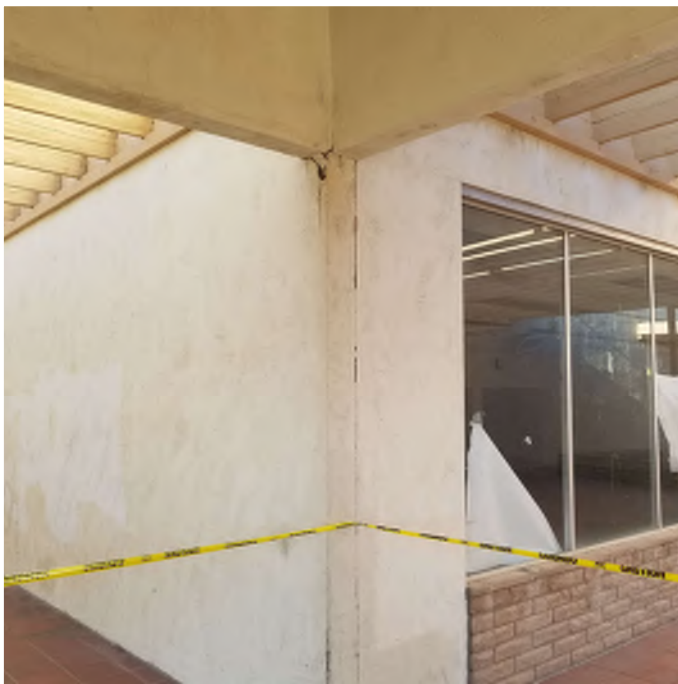
Photo K - Crack on facade
