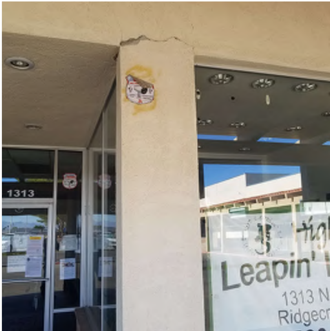
Photo I - Crack on facade
