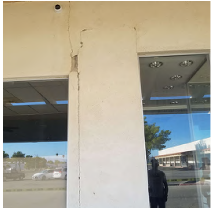
Photo J - Crack on facade
