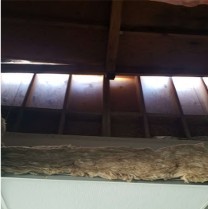
Photo Q - Roof detached from exterior wall
