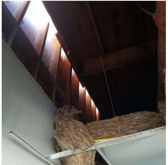
Photo P - Roof partially collapsed inside of the leaning wall
